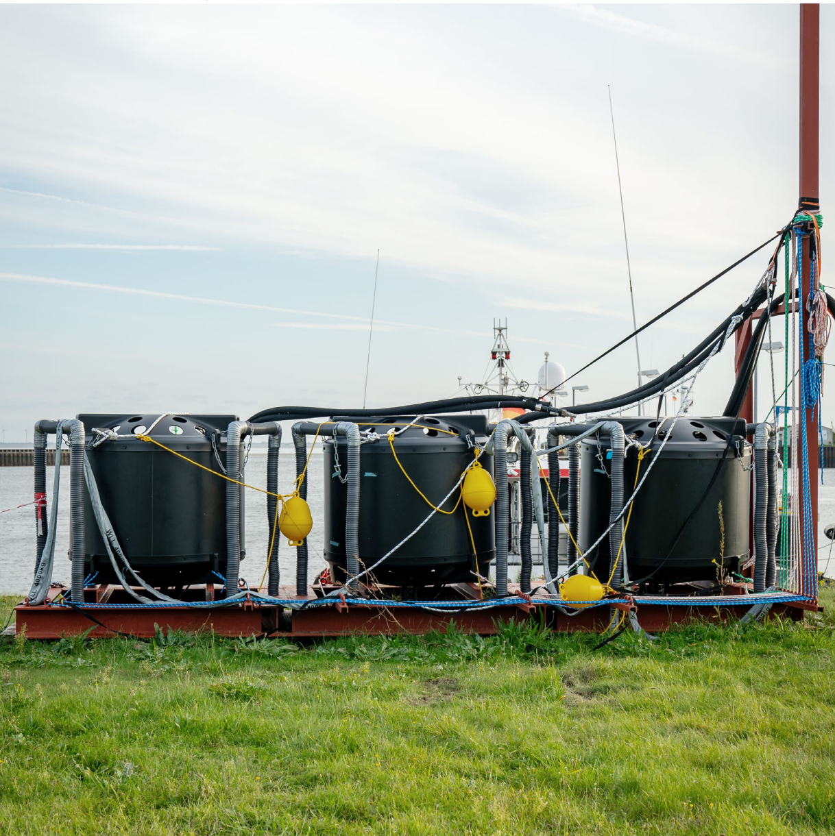
Germany's first seawater source heat exchanger was installed in Borkum's harbour this summer © Nordseeheilbad Borkum GmbH
